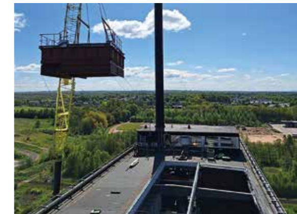
The Scheuch solution was implemented in the existing building.
