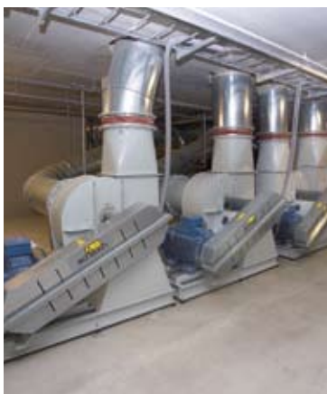
Transport fans for group extraction system
