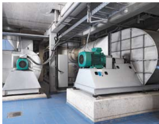
Fans with coupling drive
