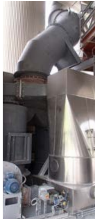
Partly visible cyclones for separation of the heated dust particles after the thermal treatment in the second preheater line
