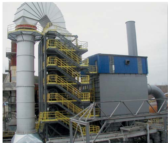
Figure 7: Air/air heat exchanger and EMC filter plant at the Malogoszcz cement works in Poland
