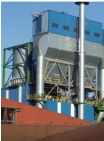
Pressure surge resistant filter for dedusting a coal grinding mill
