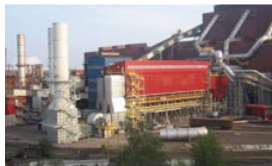
Chamber filter in the steel industry
