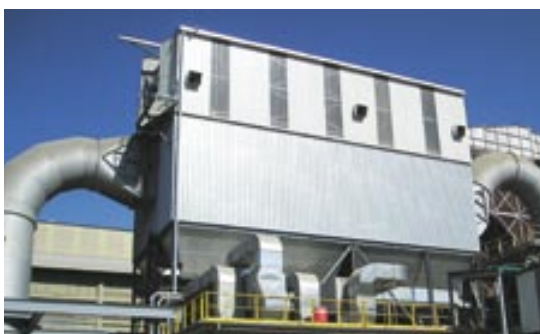
Chamber filter in the cement industry
