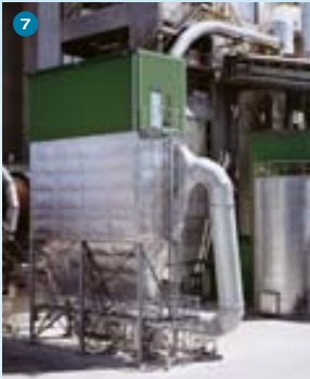
7 Chlor-Bypass-Entstaubung chlorine bypass dedusting unit
