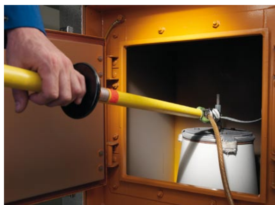
Grounding of insulator
