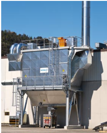
ESP with attached exhaust stack
