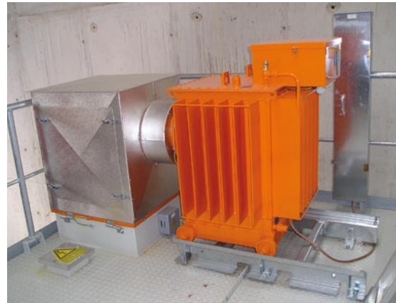
Transformer on castors
